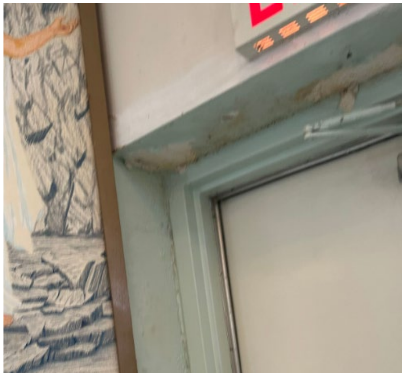
Figure 8 - Previous repair / leak at emergency exit of church
