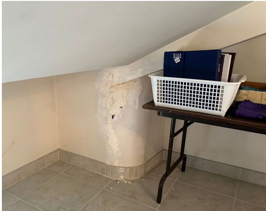
Figure 7 - Previous repair / leak in south-east corner of church
