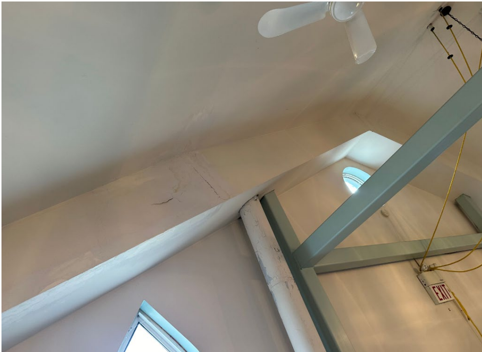
Figure 5 - Previous repair / leak on south wall of church
