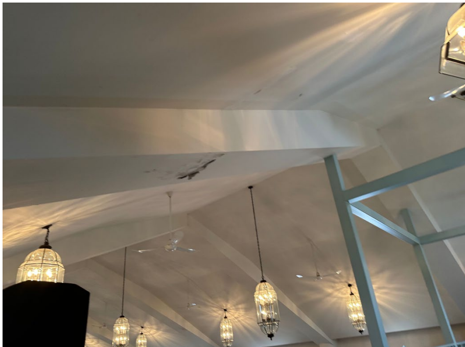
Figure 4 - Previous repair / leak in south-west corner of church
