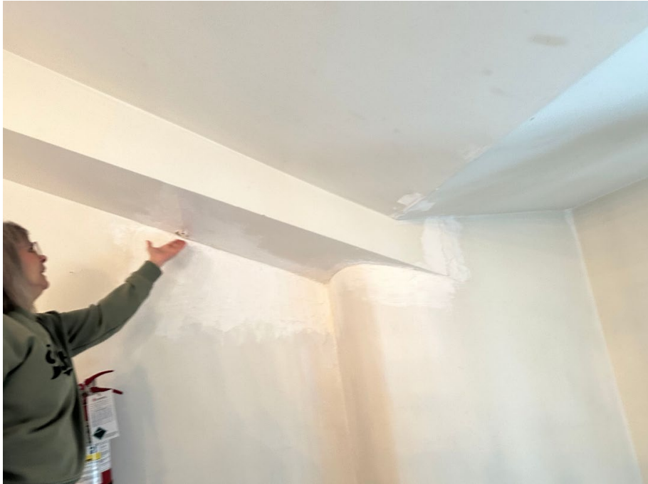
Figure 3 - Previous repair / leak in south-east corner of church
