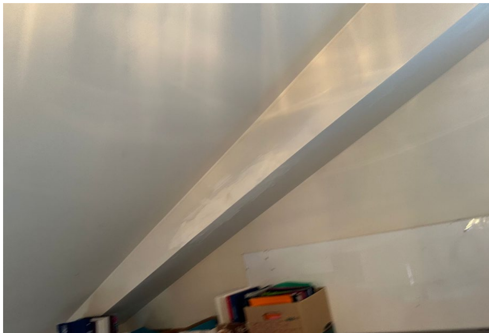
Figure 6 - Previous repair / leak on south wall of church
